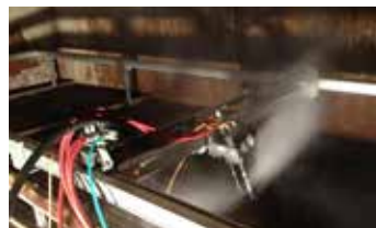
CONDENSER TUBE CLEANING
